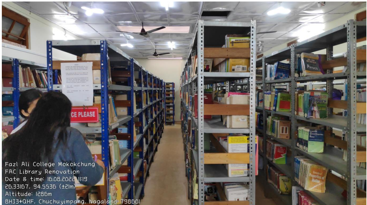
Fazl Ali College Mokokchung FAC Library Renovation Date & time: 16.08.2022 11:19 26.33175, 94.55355 (±8m) Altitude: 1286m 8HJ3+QHF, Chuchuyimpang, Nagaland 798601
